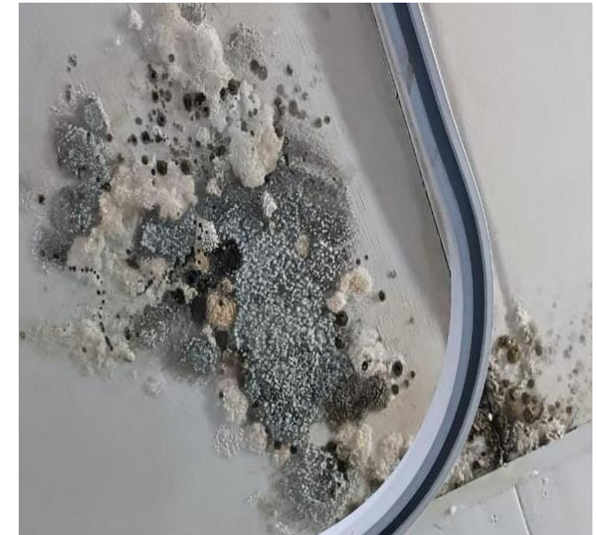
Fungal growth over roof
